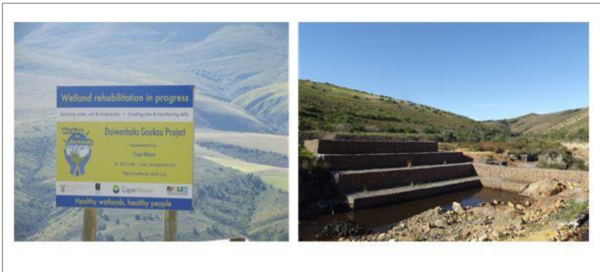
Figure 24: Duiwenhoks Goukou Wetland Rehabilitation Project adaptation mechanism. Top left; signpost positioned to inform public of on-going conservation programmes at Duiwenhoks catchment; top right; gabion structure in process of construction during the study site visit (16 July 2014).
